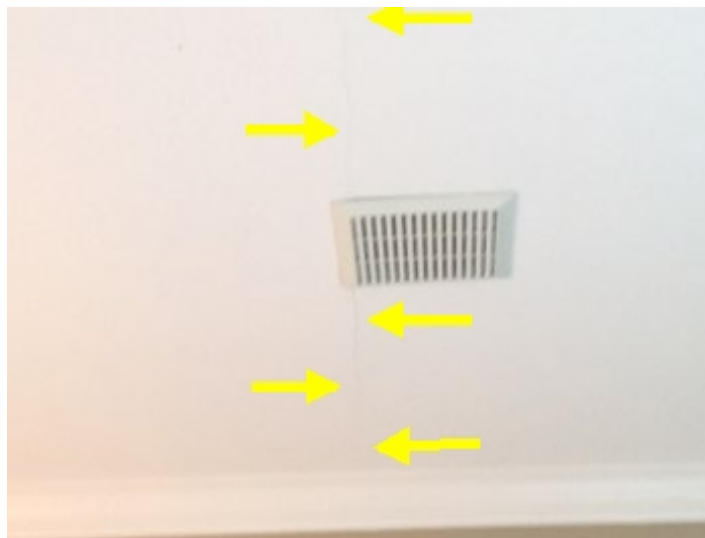
Crack in master bathroom ceiling. Cosmetic
