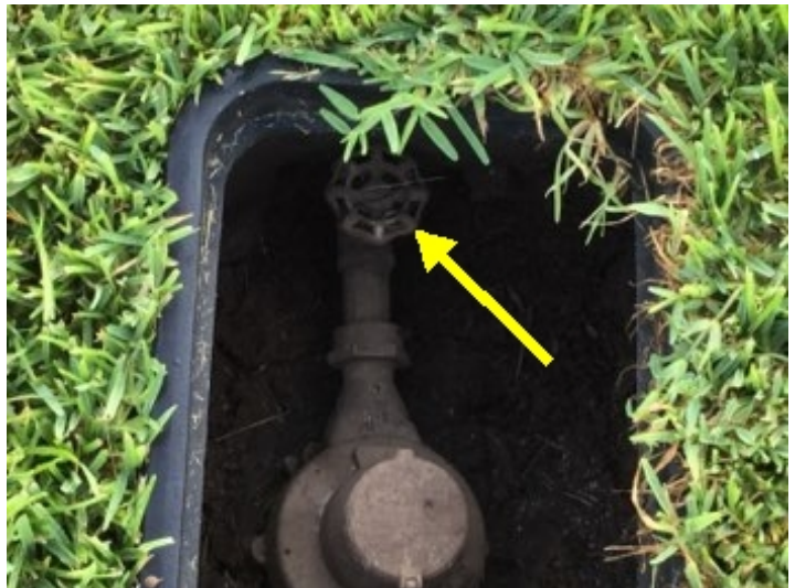
Water cut off valve for house
