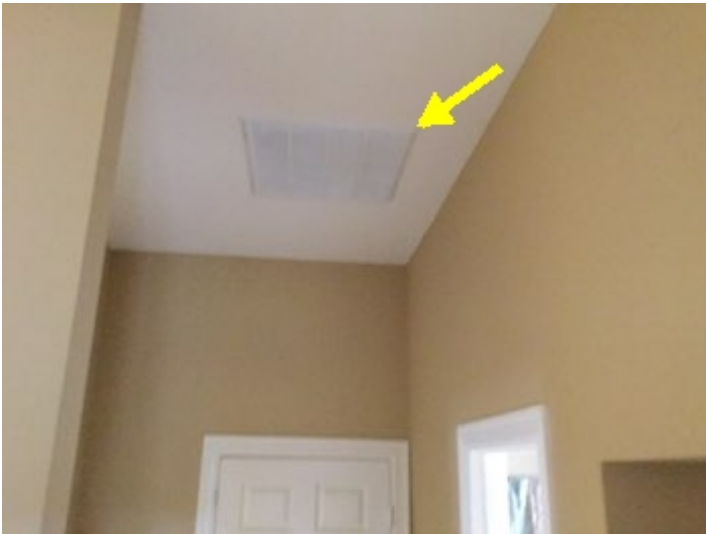
Return air grill in hallway ceiling by stairway. 20 X 20 filter
