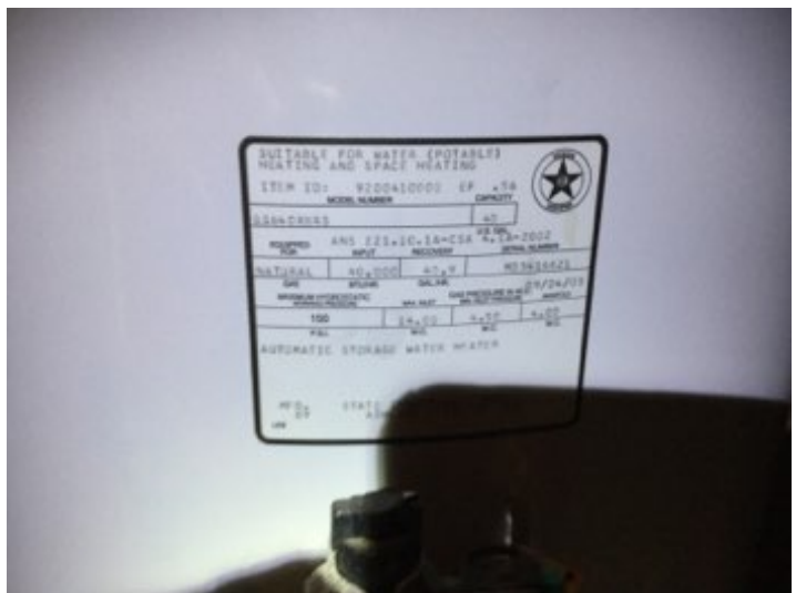
Water heater data plate #2
