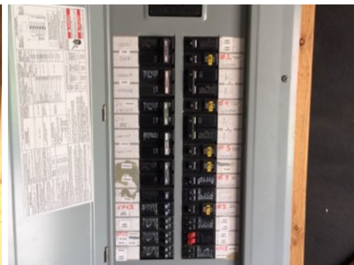
Panel is properly marked
