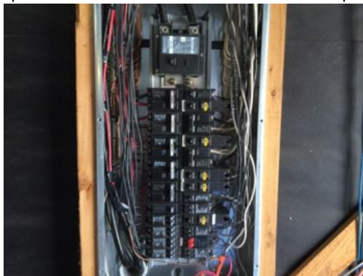
Interior of breaker panel
