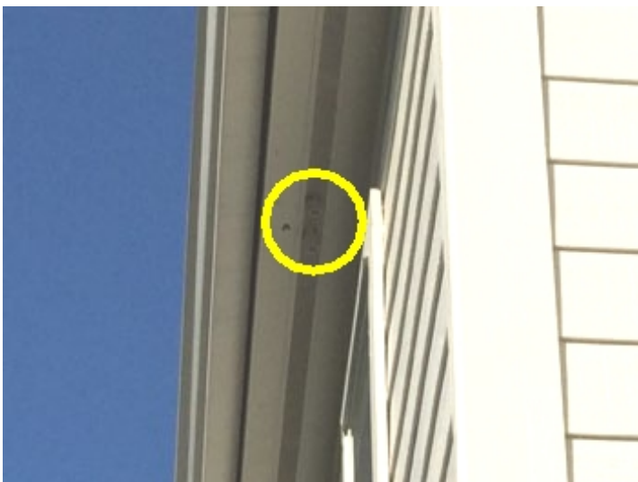
HVAC system evaporator coils secondary drain lines
