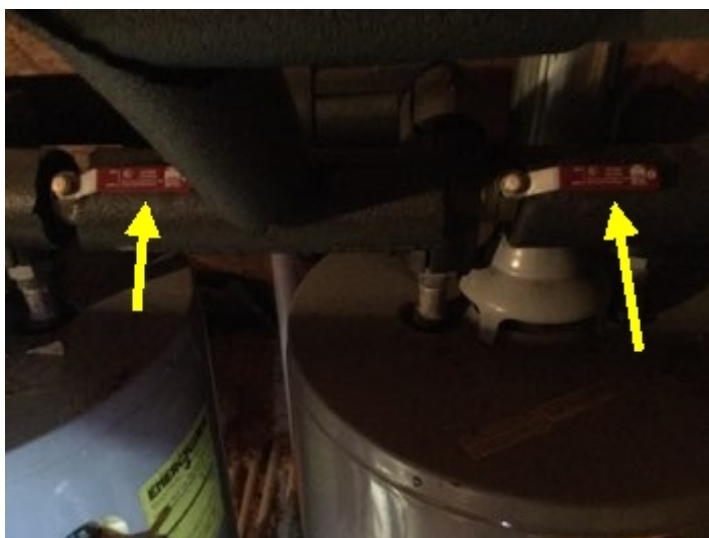
Water heater cut off valves
