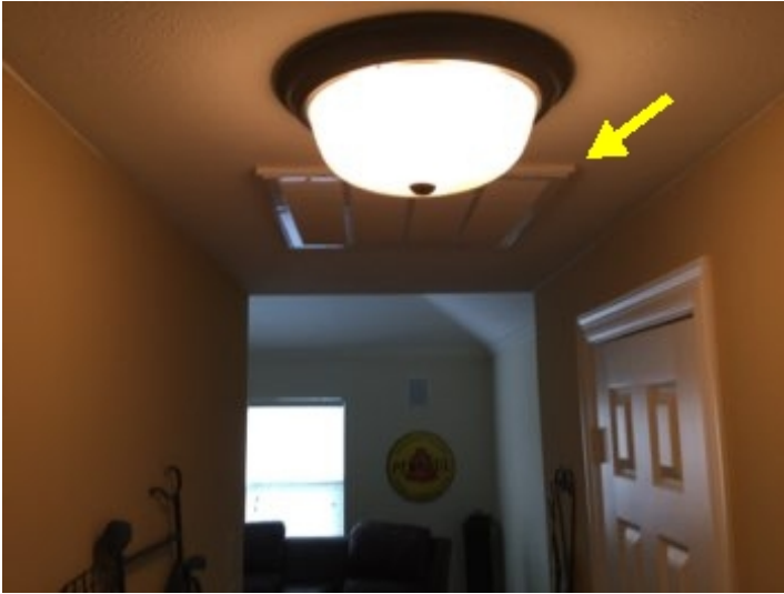
Return air grill located in hall ceiling going to media room. 20 X 20 filter
