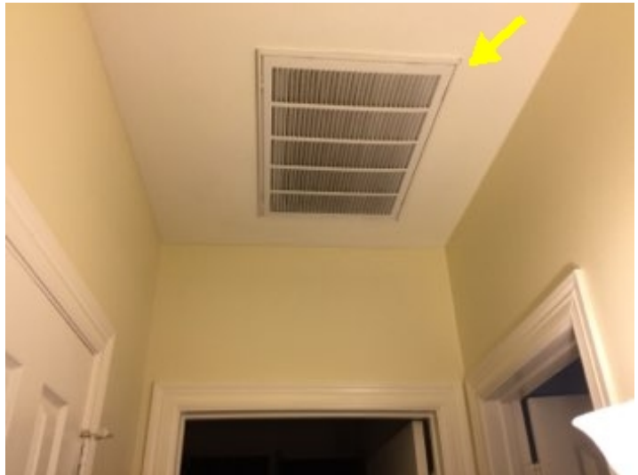
Downstairs return air grill. 16 X 20 filter
