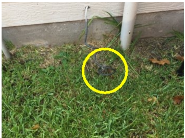
Ground rod for electrical system
